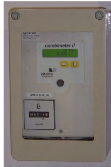
Meter for solar water heating system
